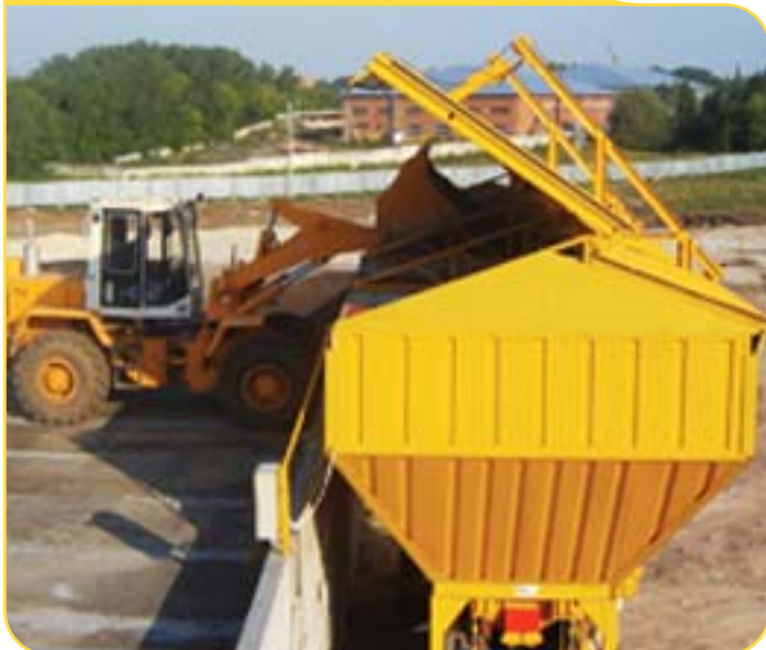
Aggregate Inline Silo
